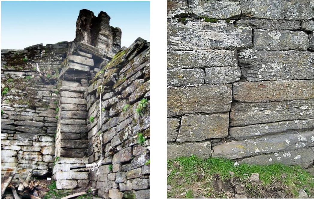
Figure 4. Earthquake jostling in Šarda Complex a. joint of stair case with the main court b. outside view of the base of the northern wall
