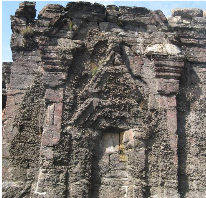
Figure 6. Deteriorations caused by biological growth on the surface
