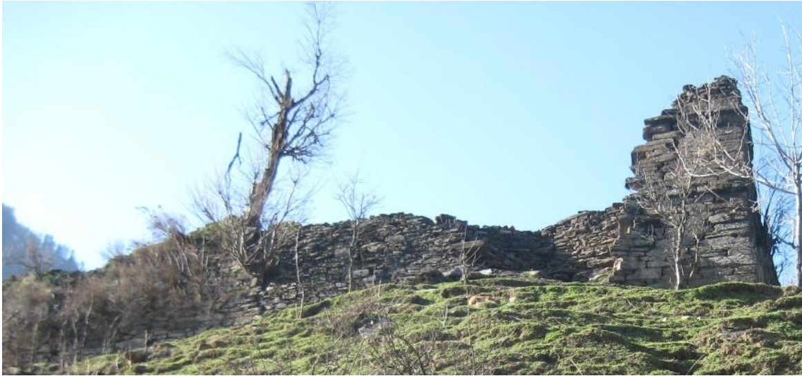
Figure 1. Southern side of the temple lapsed due to the weakening of foundations by floods
