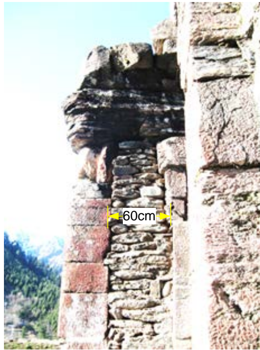
Figure 14. The remaining pillar of the canopy to the door from southern side in front of door. These repairs have cement used in some instances.
